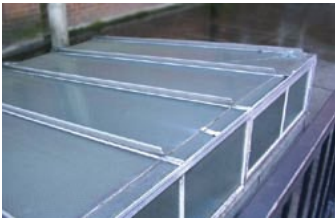
Chrysotile string on skylights
