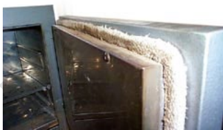
Asbestos rope seal on drying oven
