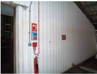
Chrysotile/bitumen coating under metal cladding
