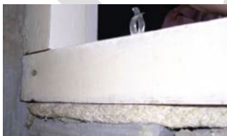
Amosite asbestos rope packing on riser door frame
