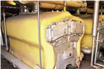
Amosite lagged boiler with vessel hard plastic coating
