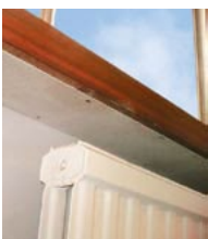
AIB panel between radiator and window
