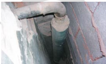
Lagged pipe in wall cavity
