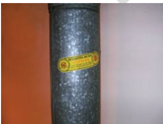
Metal clad gas flue containing chrysotile lining
