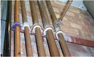
Chrysotile cloth on pipes
