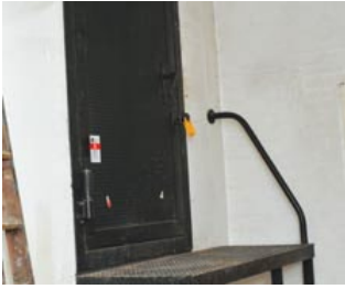
Composite steel and asbestos fire door
