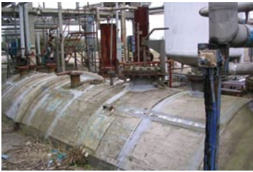
Lagging on large petrochemical plant
