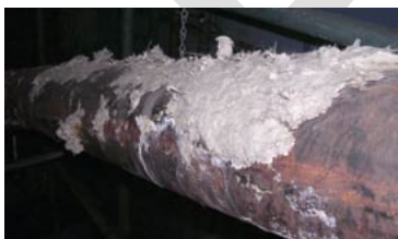
Amosite lagging in very poor condition on steam pipe
