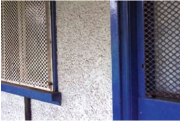
Chrysotile pebble-dash exterior wall coating
