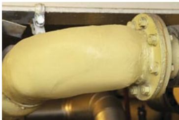
Pipe insulation with coating in a passageway
