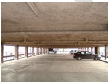
Sprayed limpet on car park roof
