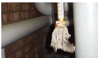
Asbestos rope lagging to boiler thermometer
