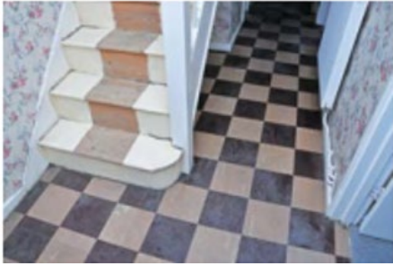
Asbestos-containing vinyl floor tiles
