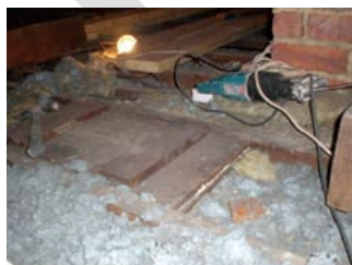
Loose asbestos used as loft insulation
