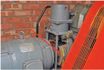
Asbestos brake lining on output shaft of AC motor
