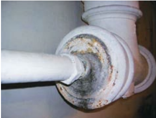
Amosite and chrysotile packing on waste pipes
