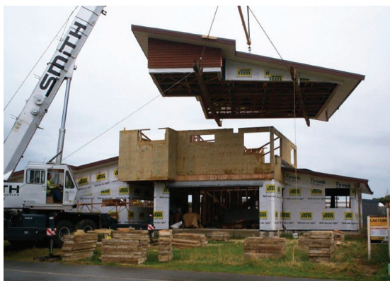
Figure 1: Craning a pre-assembled roof into position greatly reduces the need for work at height (Image courtesy of BJ Carter.)
