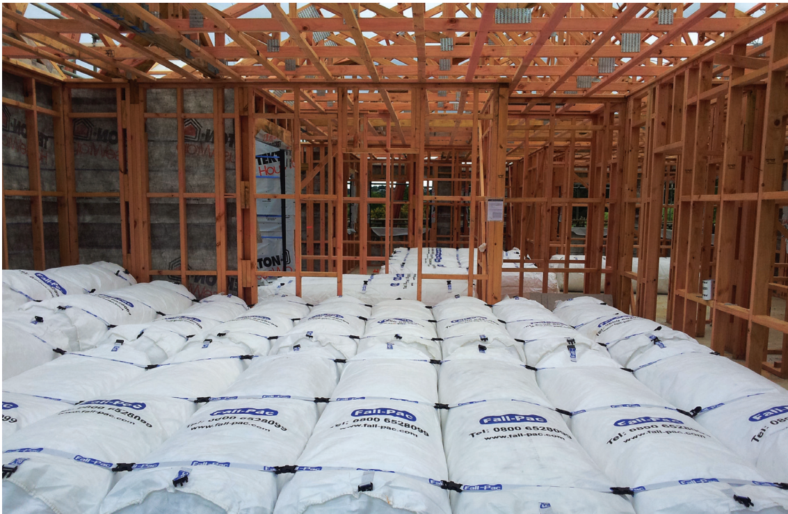
Figure 7: Bean bags being used as a fall mitigation measure during roof work (Image courtesy of Fall-Pac NZ Limited).
