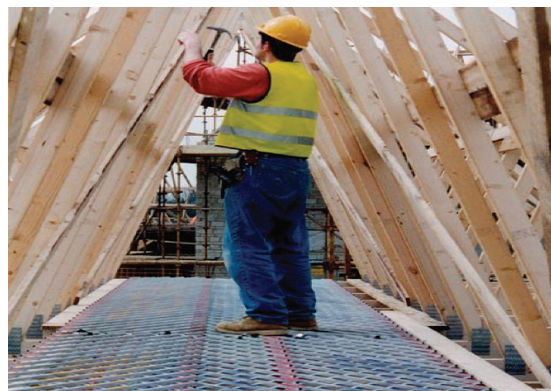
Figure 2: Decking system that provides a working platform in the roof eaves (Image courtesy of Oxford Safety Components Ltd).
