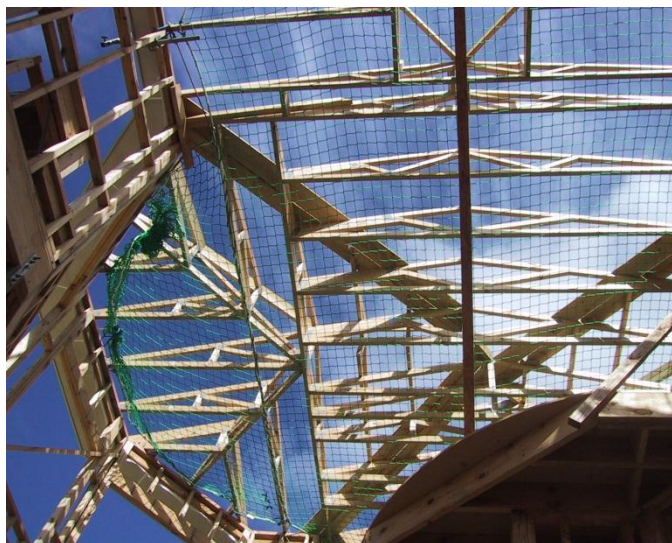
Figure 6: Safety nets set up under a roofing construction to catch falling workers, debris, or tools.
